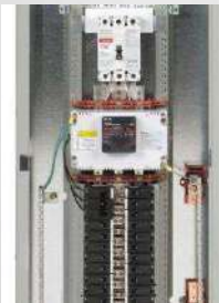
Wired connection through a breaker Better than side mount
